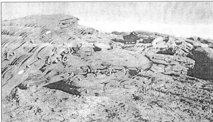
These are blasting mats. They are used when the shots come near buildings to control flying rocks. They are overlapped like shingles over the blast site.
