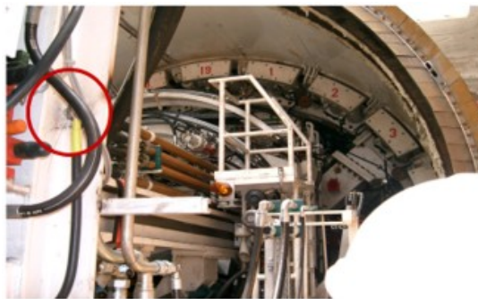
Figure-7: Connection of the measuring electrode A0 (INTEGRAL mode) near cutter head.
