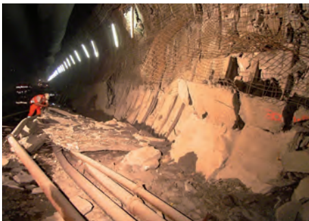
Figure 17 : Unforeseen ground conditions due to rock burst phenomena® ATG
