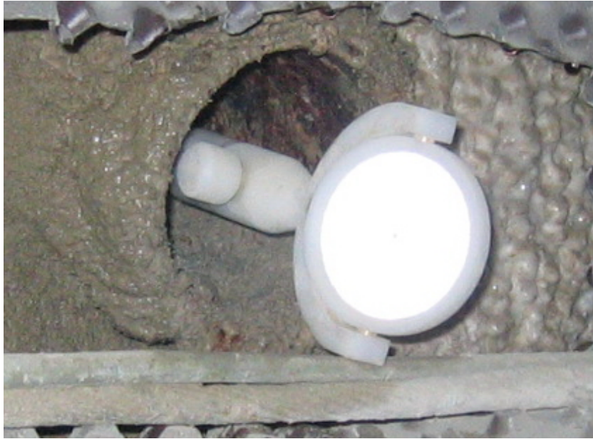
Fig. 19: Example of monitoring target with protection pipe to avoid damage of the bolt
