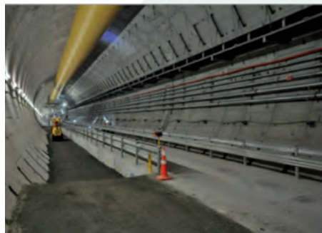
Figure 3 : Top right: Pipe-jacking tunnel as water sewer Lower right: Backfilling the gaps aside of an invert gallery in a large tunnel parallel to tunnel excavation © Babendererde Engineers
