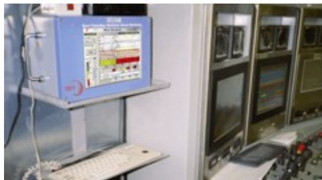
Figure-9: BEAM Unit in operator cabin
