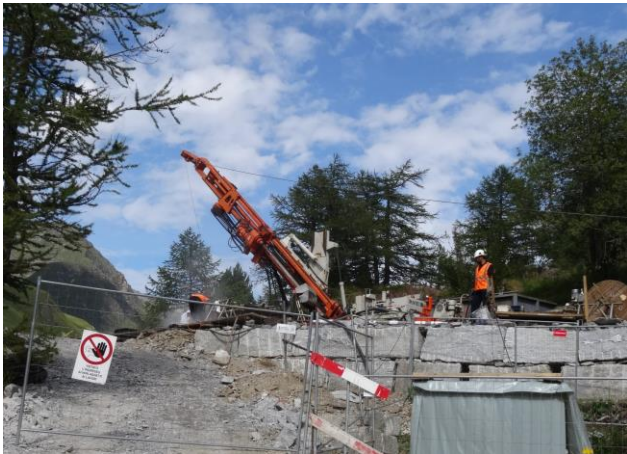
Exploratory drilling SB-05 in Piora Inclined drilling L = 750 m for an exact determination of the geological and hydrogeological conditions in the inclined shaft
