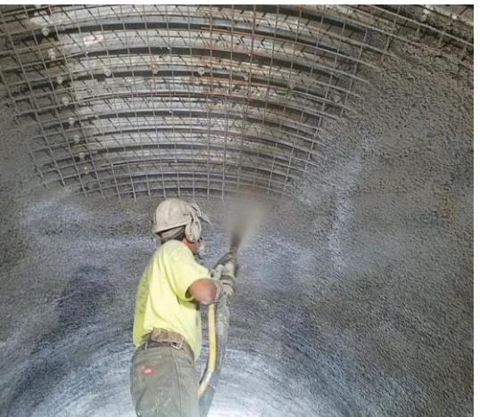
Overhead application of silica-fume shotcrete. Because of its increased cohesion, silica fume shotcrete has much less rebound and allows for greater lift thickness when shooting overhead than shotcrete without silica fume.
