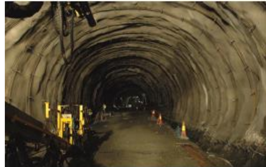
Figures: Execution of RRS in a tunnel in Oslo (Grimstad et al, 2003 and NPRA, 2010)
